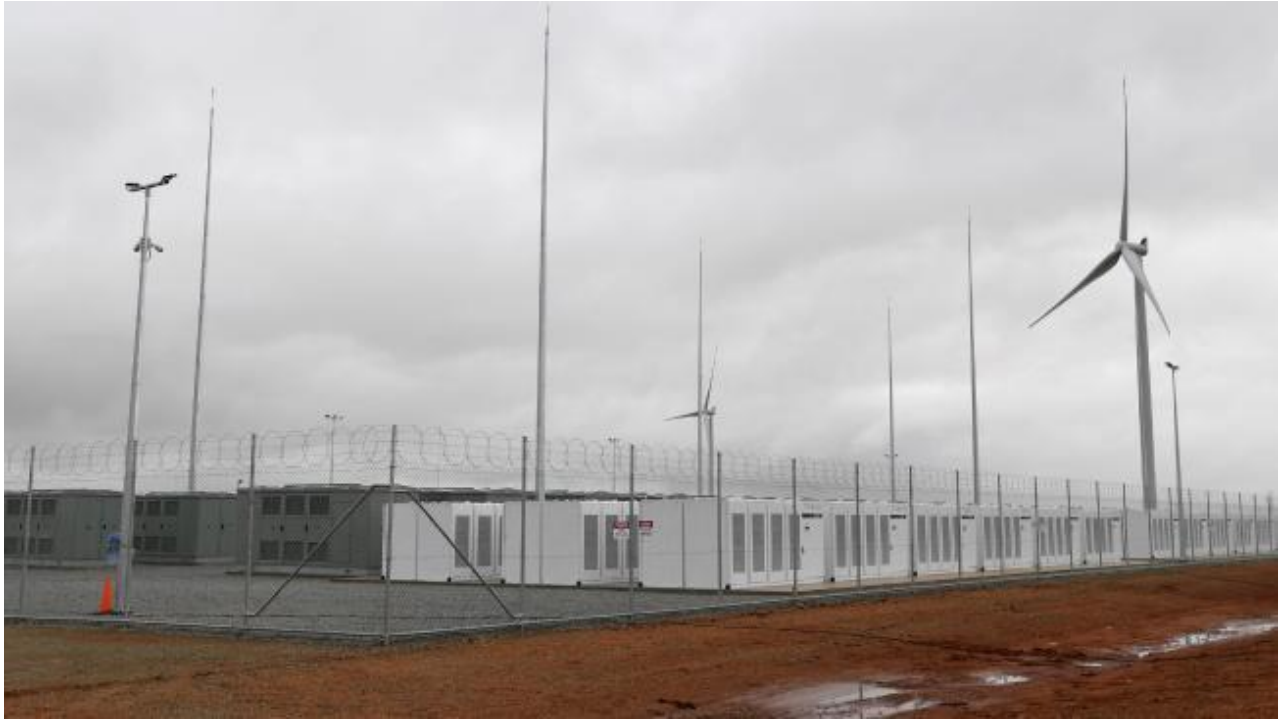
Figure 1: Jamestown Tesla battery farm, approximately 20km from Yarcowie cobalt project (source: http://www.adelaidenow.com.au/news/south-australia/worlds-largest-lithium-battery-switched-on-near-jamestown/news-story/2c4992845ce77309d7dad0d48a2d754c )
